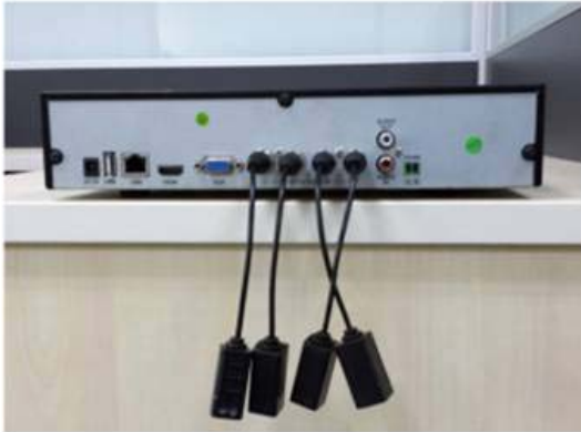
Old baluns make the cabinet a mess
